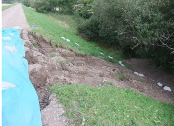
Figure 48. S-2: Erosion on slope of dam body
