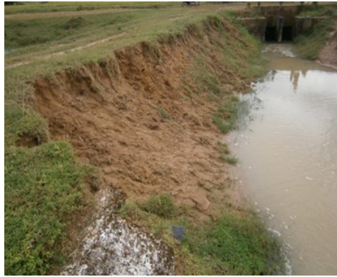
Figure 64. S-2: Significant erosion on canal
