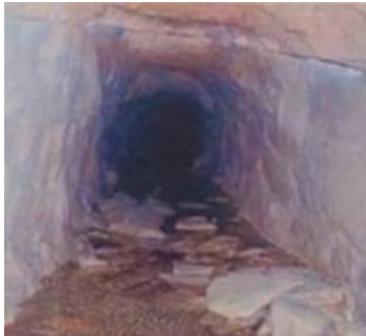
Figure 56. S-2: Significant breakage on concrete lining on conduit
