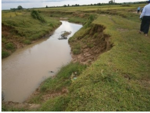
Figure 63. S-3: Erosion on canal
