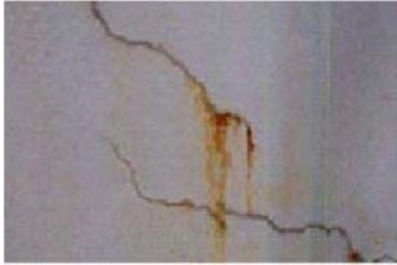
Figure 57. S-3: Cracks and corrosion of rebar inside of concrete
