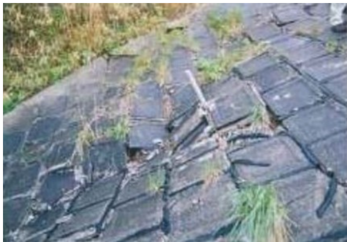
Figure 50. S-3: Breakage on slope protection of dam body
