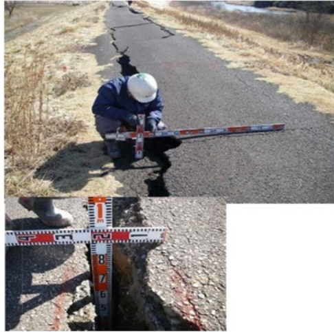
Figure 46. S-2: Big and long cracks on top of dam body
