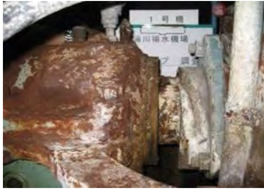
Figure 69. S-2: Significant corrosion on bearings of pump motor
