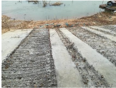
Figure 4. Improper steel work
