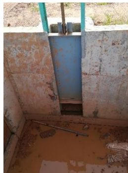
Figure 5. Cracks on water gate
