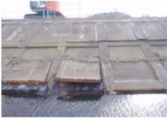
Figure 54. S-3: Breakage on revetment
