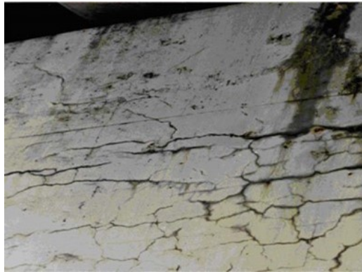
Figure 58. S-3: Alkali silica reaction on concrete
