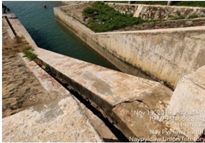
Figure 52. S-3: Crack on headworks spillway
