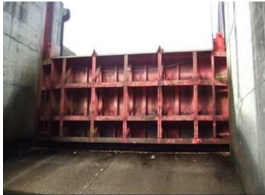
Figure 59. S-3: Rusting gate
