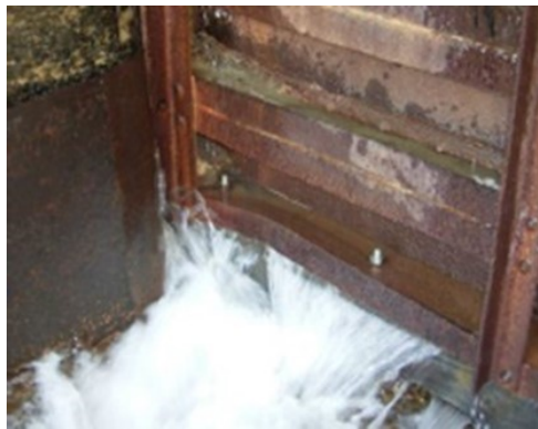
Figure 62. S-2: Water leak from gate
