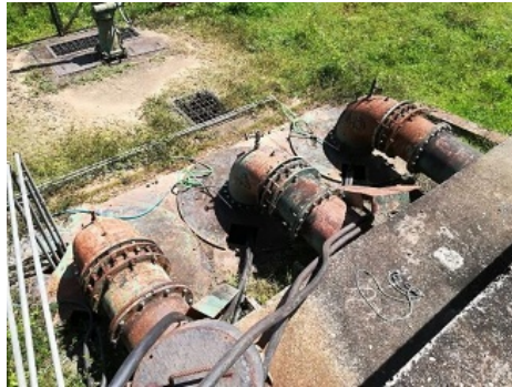
Figure 3. Rusted pipes of irrigation pump
