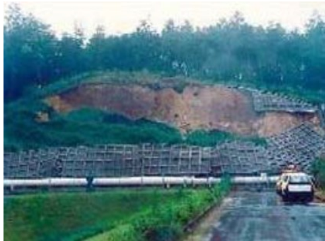
Figure 49. S-1: Collapse of slope protection of dam reservoir
