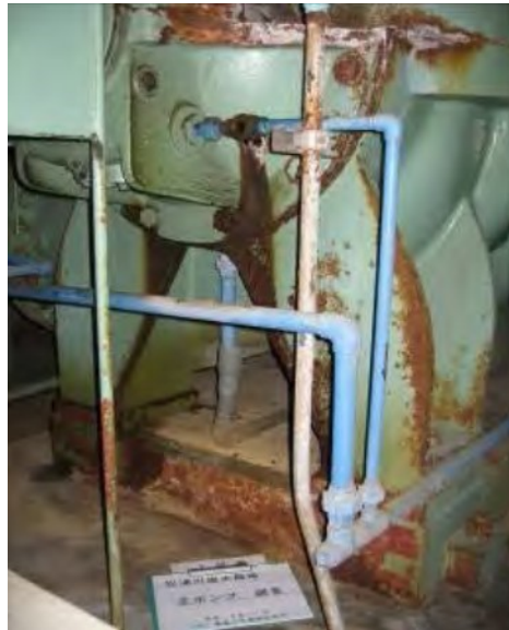
Figure 68. S-3: Rust on bearings of pump motor
