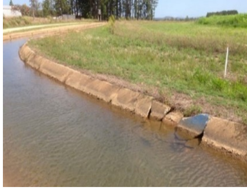
Figure 66. S-3: Breakage of concrete canal lining
