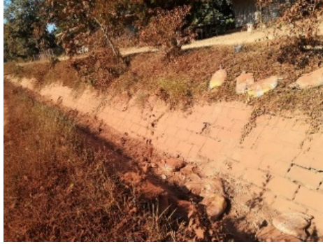
Figure 1. Cracks on canal wall
