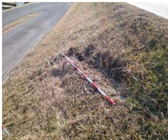
Figure 47. S-3: Hollow on slope of dam body
