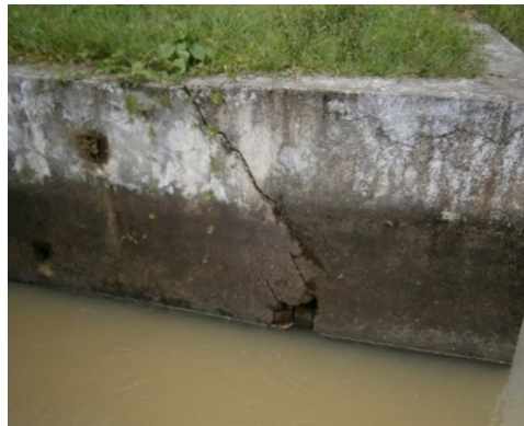
Figure 67. S-3: Crack on concrete water canal
