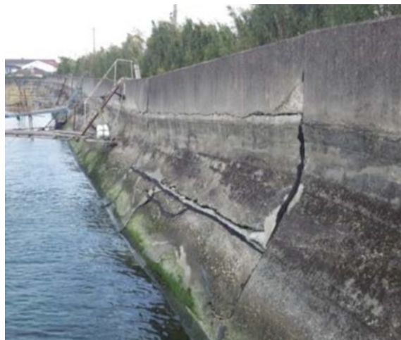
Figure 53. S-2: Big and long cracks on revetment
