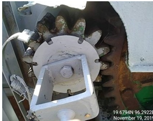
Figure 61. S-3: Rusting hoist of sluice gate
