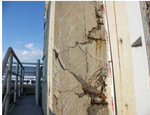
Figure 55. S-2: Significant breakage of reinforced concrete structure
