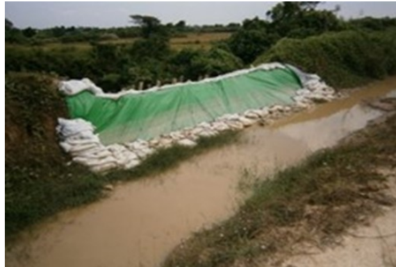
Figure 65. S-1: Collapse of canal embankment
