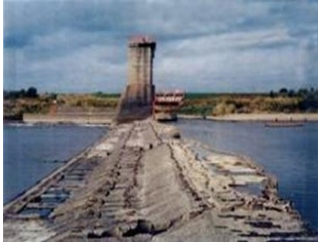
Figure 51. S-1: Collapsed headworks
